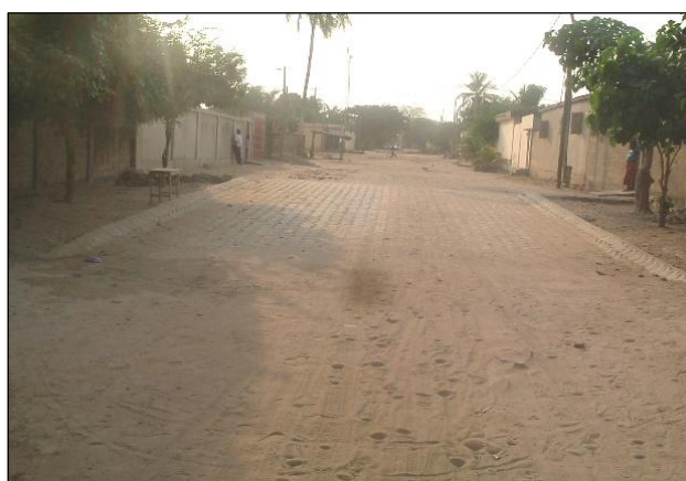
Figure 9. Work after 15 years of exploitation (2018)
